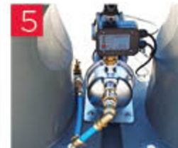
5 Pump installed with rain/mains changeover (sits behind door)
